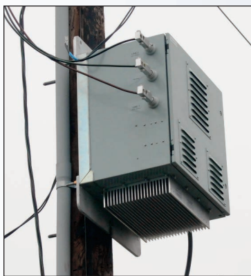
FIGURE 3: GridBridge Grid Energy Router mounted on power pole
